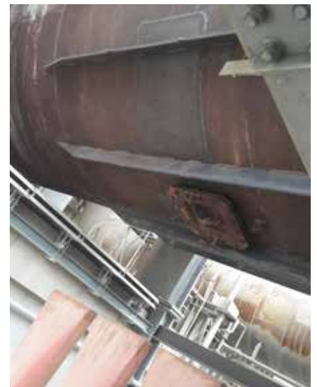
Kiln crack repair
